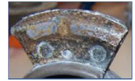
Corroded detent plate and rivets
